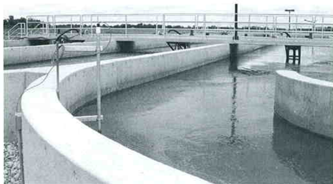
A closer view of the DO probe location on the west side of the oxidation ditch and the bridge mounted process aerator/mixer units.
